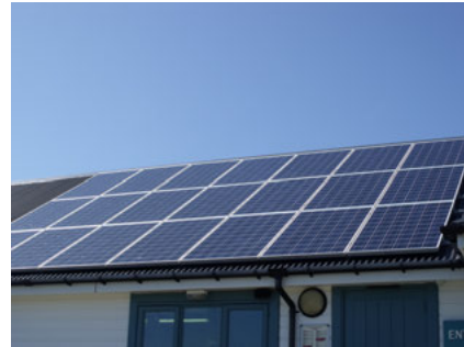
Figure 12.1: The use of solar cells to supply electricity.
